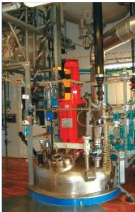
Low temperature reactor at RohnerChem
